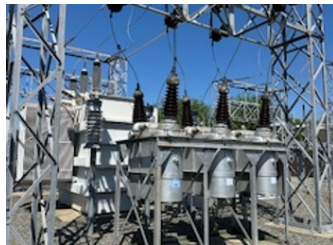
60 Kv main circuit breaker
