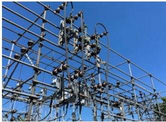
Overhead gang operated switch for making and breaking parallel between substation transformers.
