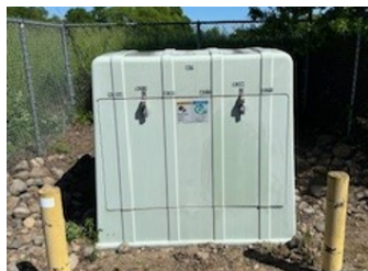
1102 underground switch cabinet
