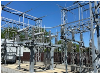
S&C 60kv main circuit breaker
