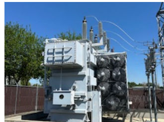
T-3 25 Mva substation transformer
