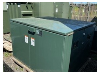
(new) 4 position gang operated underground switch
