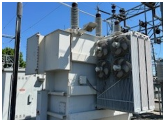
T-1 10 Mva substation transformer
