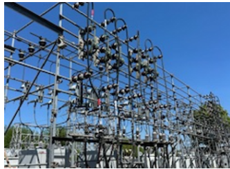
Overhead gang operated switch for making and breaking parallel between substation transformers.
